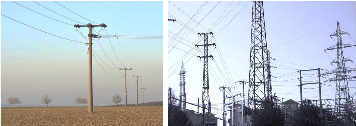
Figure 1: Examples of overhead lines with a) poles and b) lattice towers.
