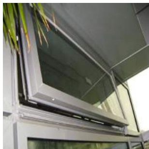
Fig. 6: Photograph of electric air shutter on 11 th floor.
